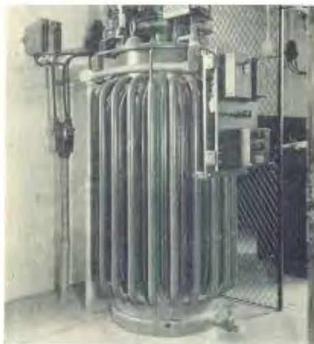
Automatic inductance regulator keeping constant the voltage on the 100-kilowatt tubes.
